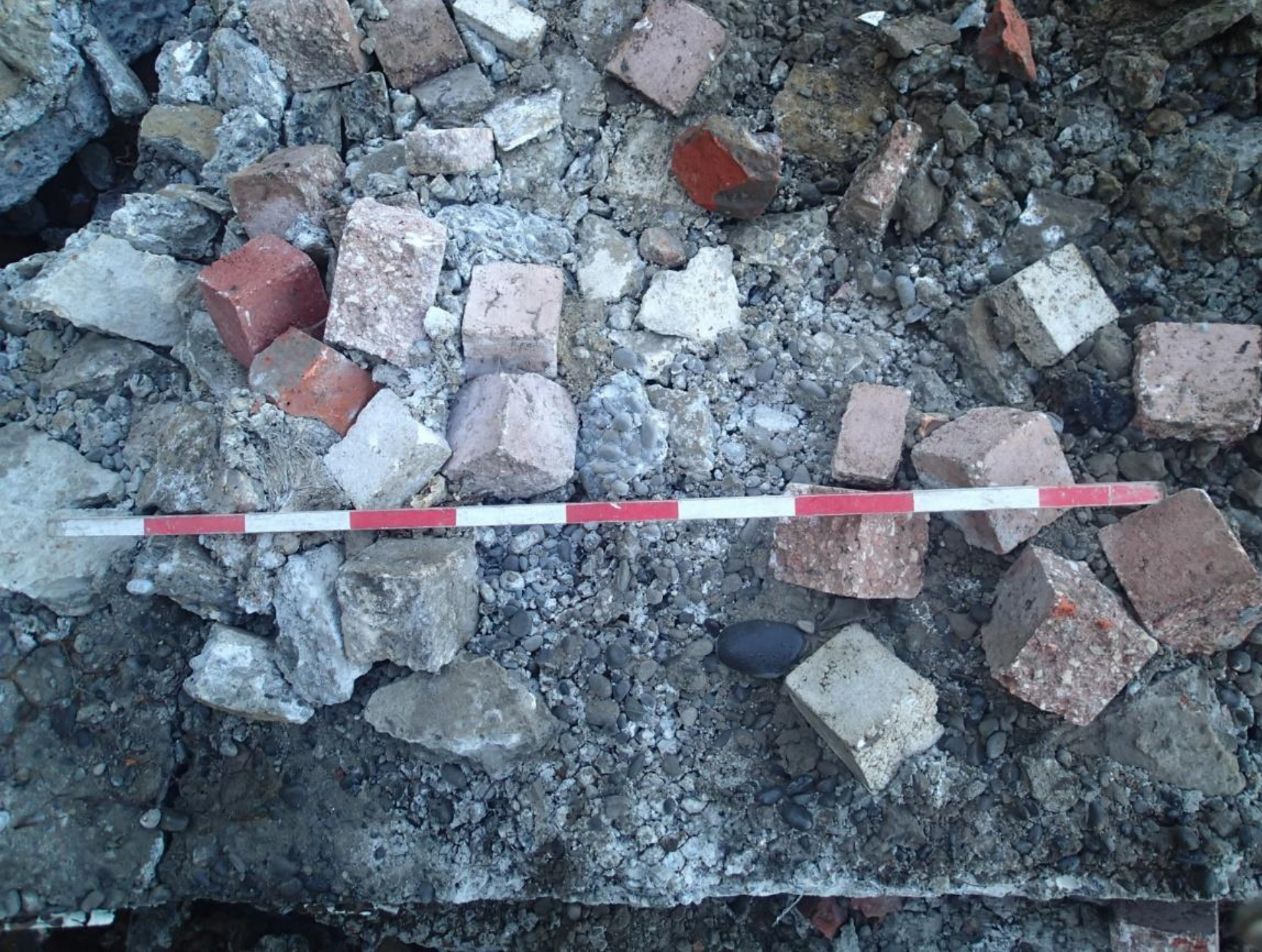
Asbestos under the patio.
