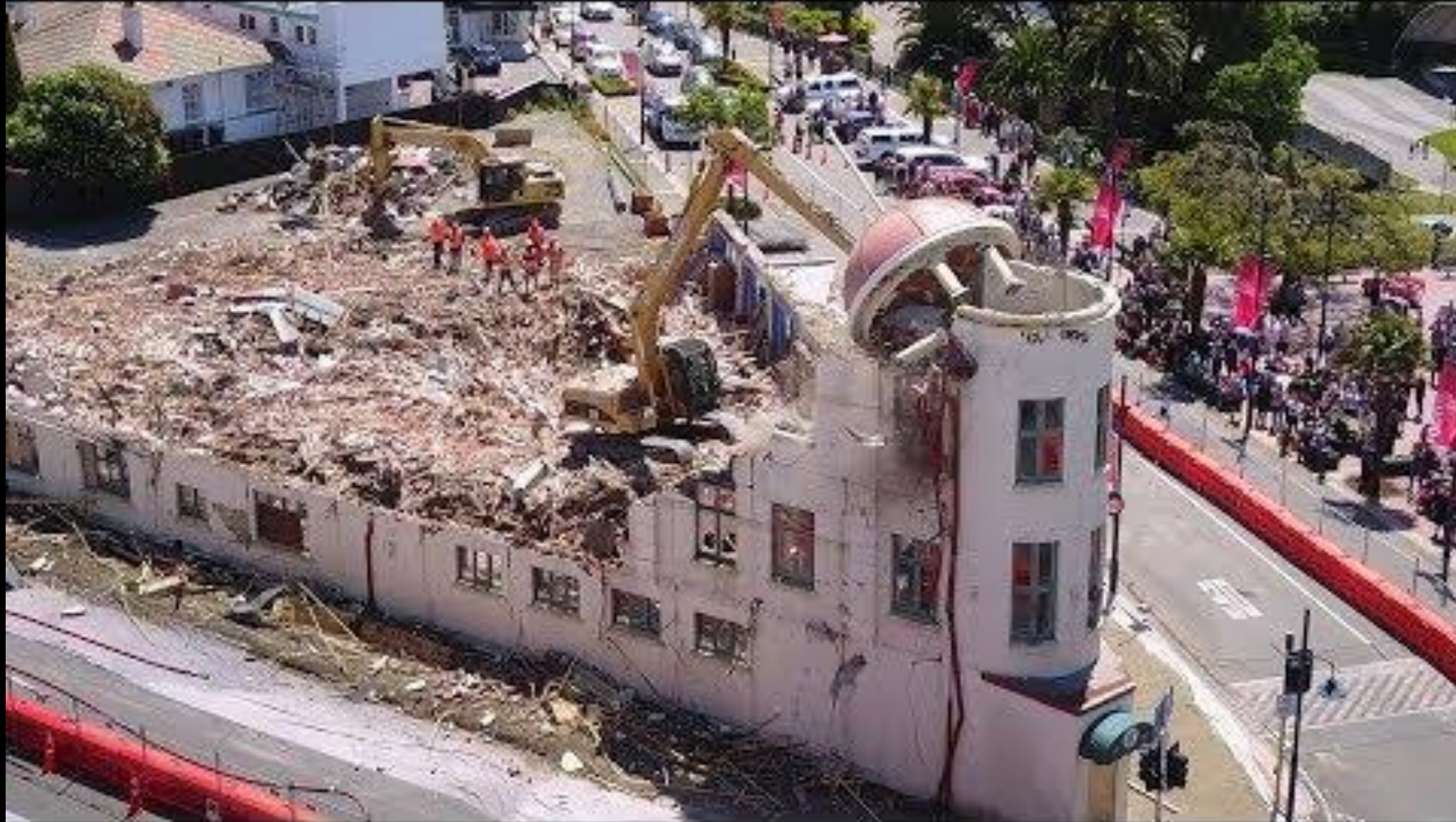
Hydro grand Hotel (1912) demolition November 2017. Uneconomic to bring building up to code
